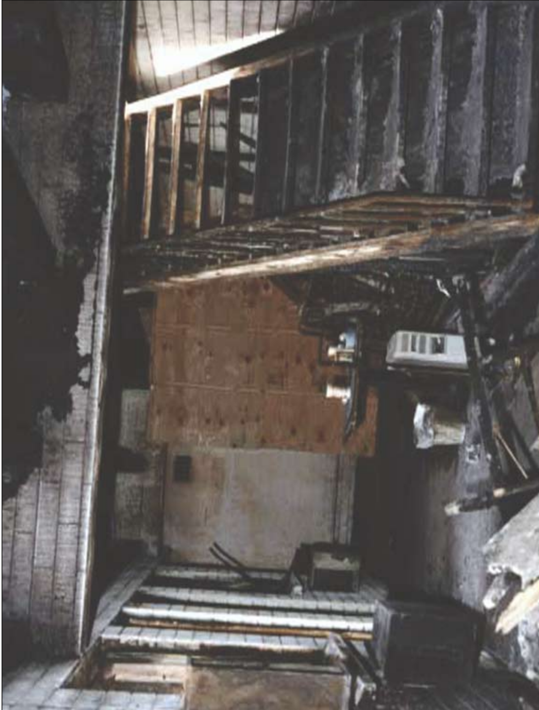
Photo 8. The 200 level breezeway area outside of Rooms 220 to 222 looking west. The open stairway to the 300 level is on the right. Under the stairs is another storage room whose wood stud and gypsum board walls were destroyed by the fire.
