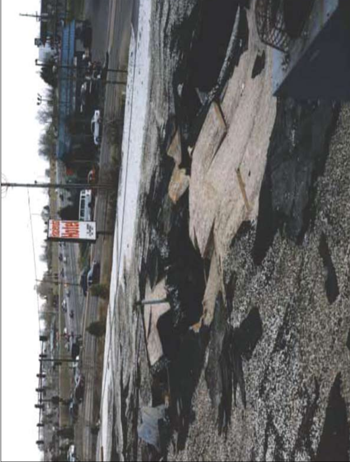
Photo 6. Roof over the front wing. The collapsed area is above the utility chase. The roof construction of Tectum board, built-up roofing, and gravel topping is illustrated.
