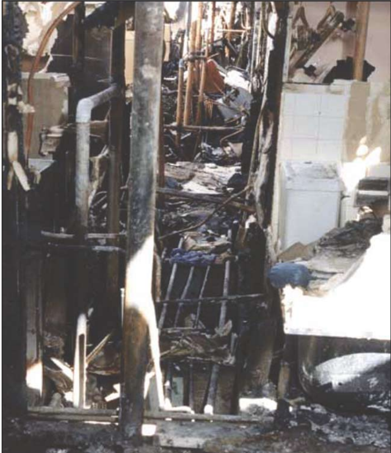
Photo 7. The west end of the utility chase in the front wing. Room 222 is to the left and Room 211 to the right. The second floor utility chase walls were burned away.
