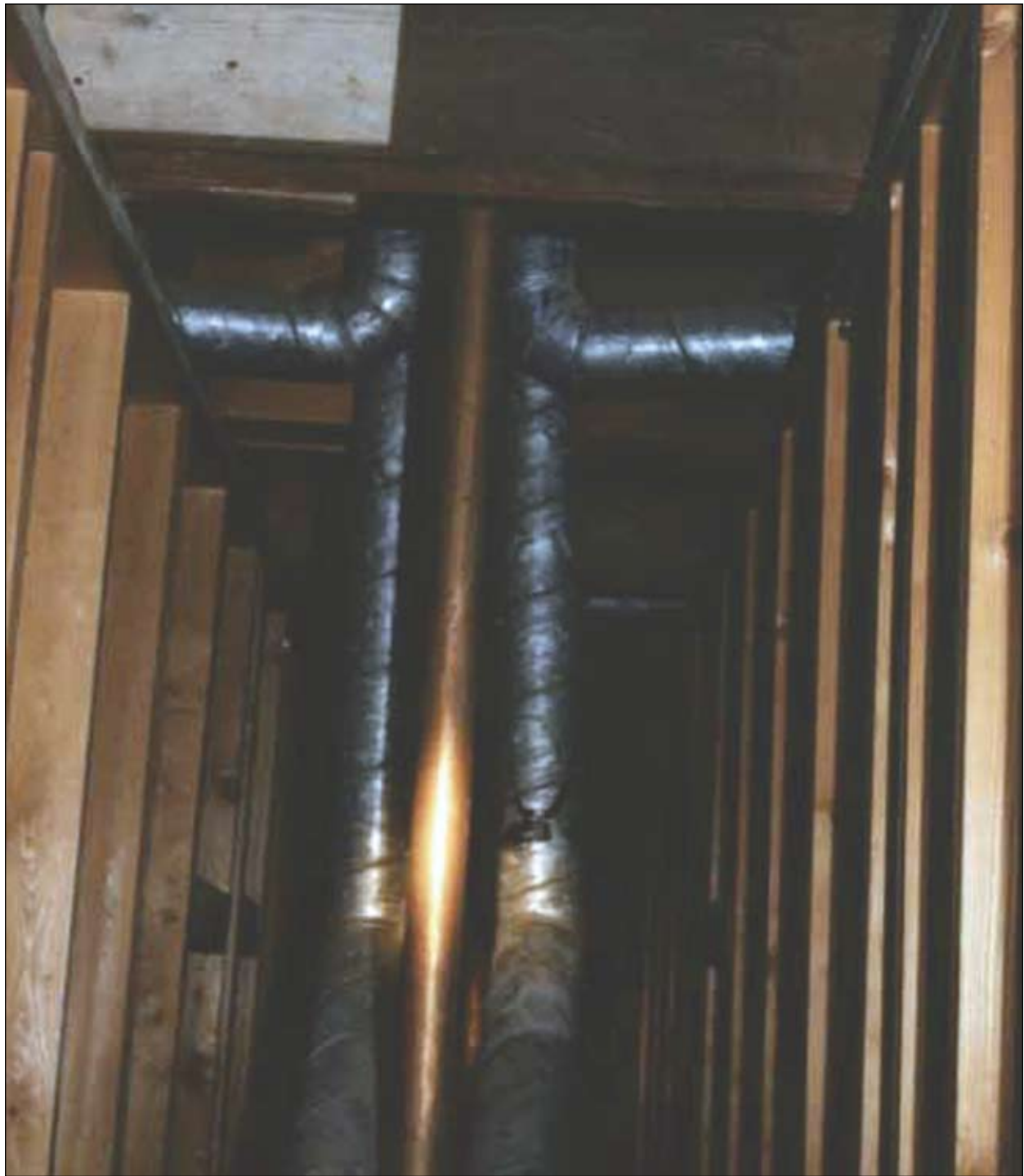
Photo 5. The interior of the utility chase between rooms showing the second floor wall construction and the wood beams supporting the roof.
