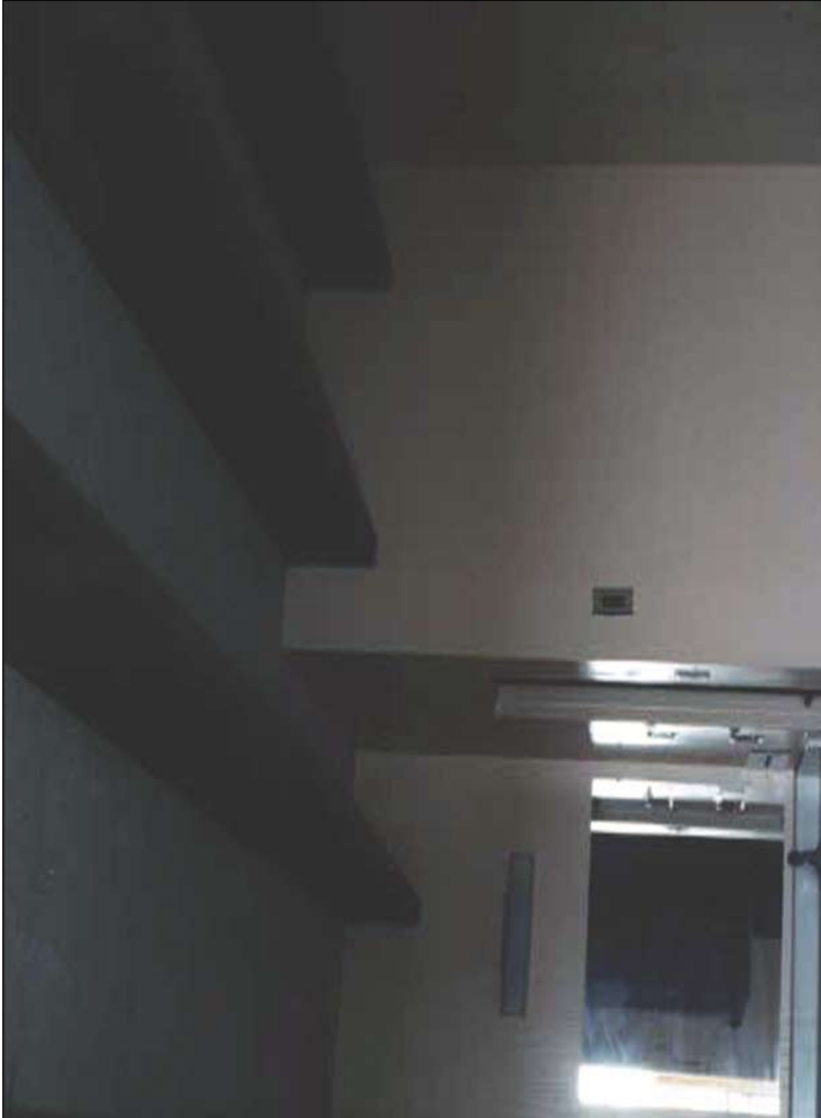
Photo 4. Typical guest room ceiling, bathroom, and sink of the utility chase wall.
