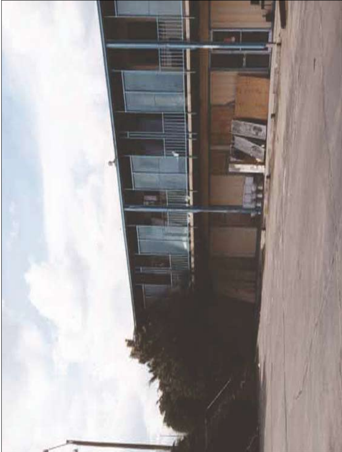
Photo 1. Southwest corner of the front wing looking northwest. The 100 level, commercial and offices, and the 200 level guest rooms are shown. The pine tree shields the entrance to the stairway and storage closet which was the point of origin.
