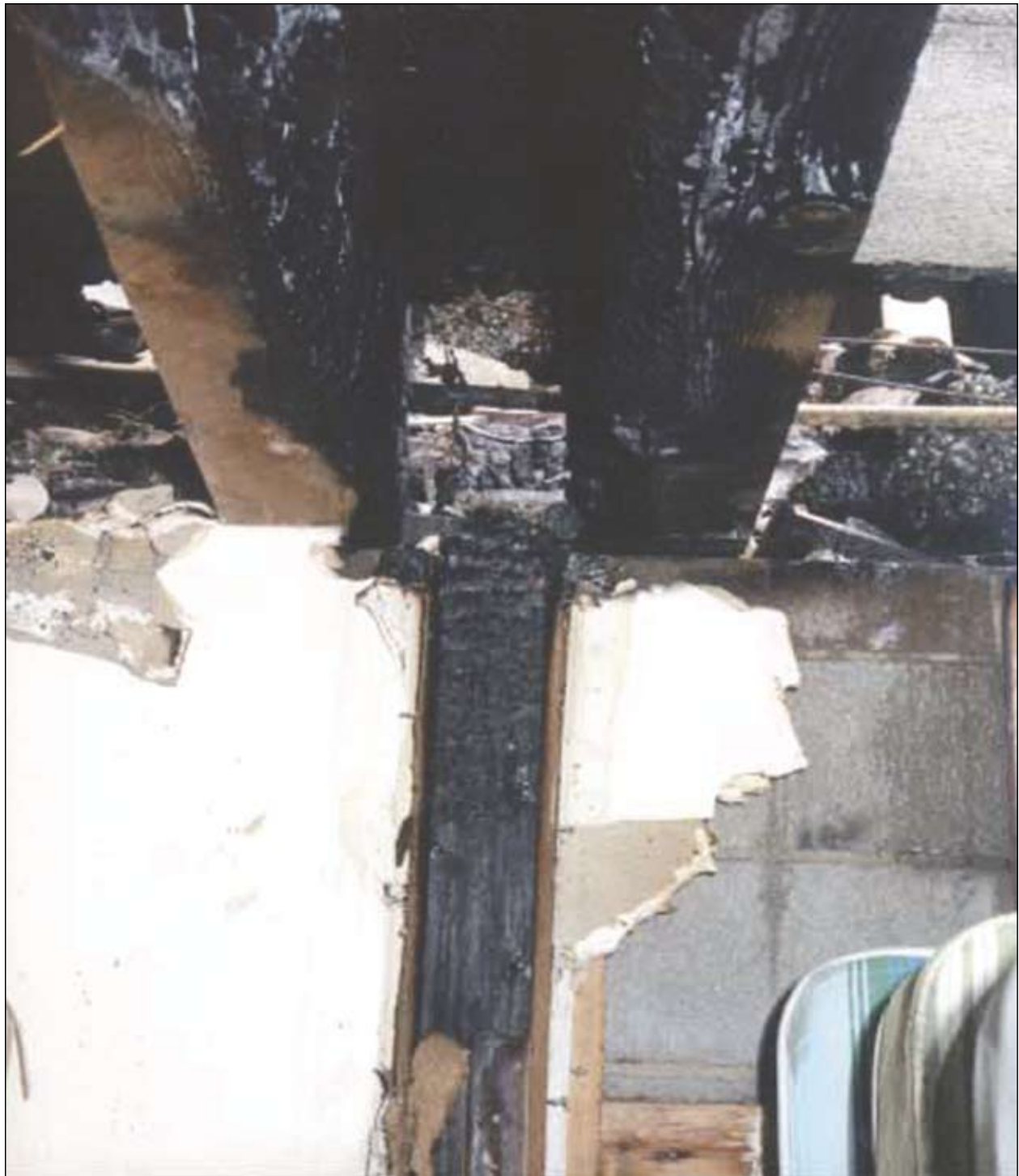
Photo 9. A separation wall between 100 level guest rooms that was burned from the inside out. The parallel wood beams formed the top of the wall and the communication to the utility chase is at the back.
