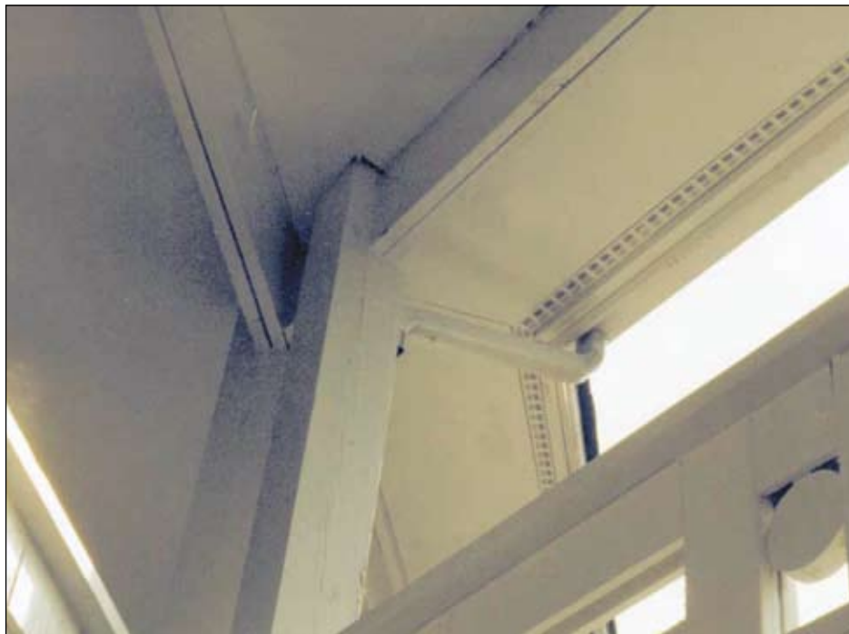
Photo 11. Typical eave line vents installed around the perimeter of the building. The fire is believed to have entered the attic through these vents.
