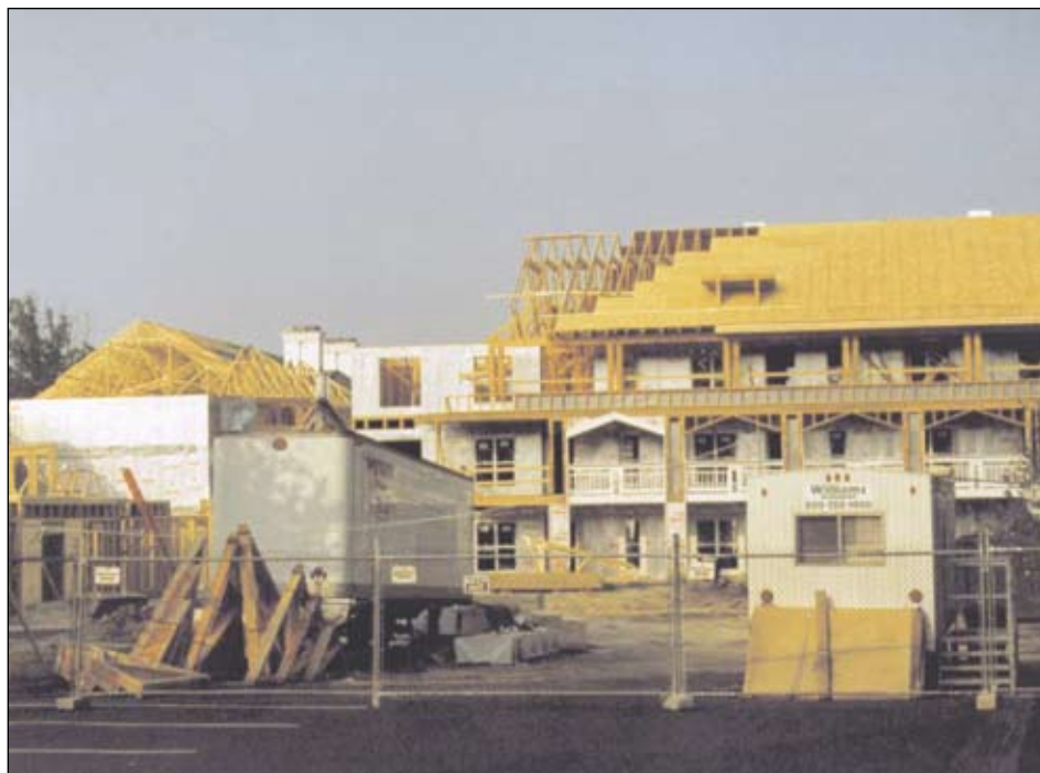
Photo 8. Reconstruction underway in Sector B, which is on the south side of the building. The exterior walkways were on the side of the wings.
