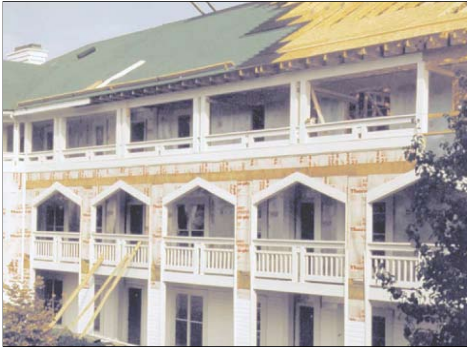
Photo 9. The exterior walkways in sector D, with the stairway located at the left edge of the photograph. The core is out of the picture to the right.
