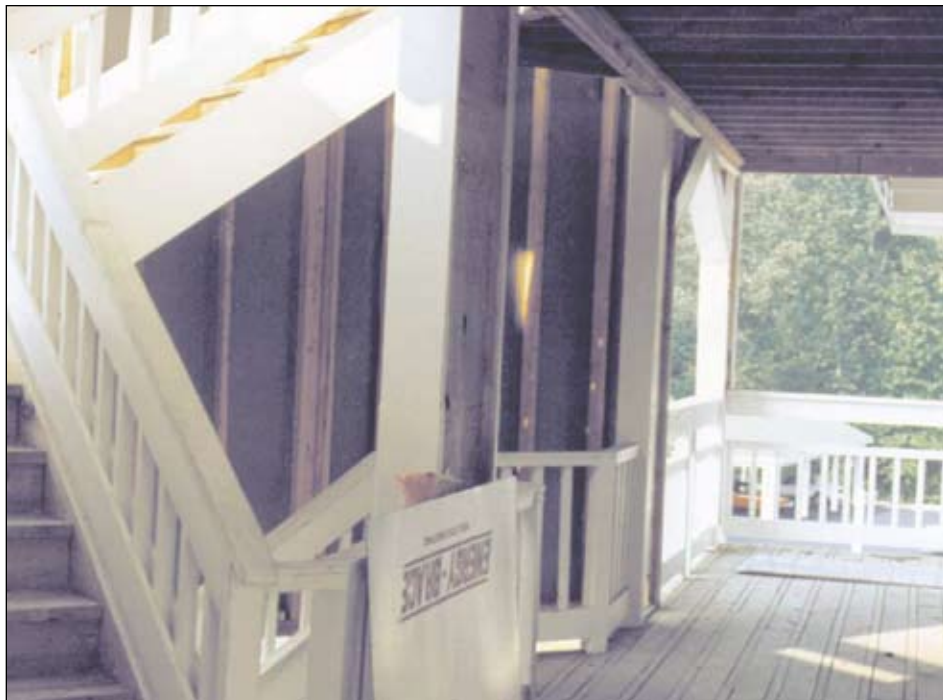
Photo 10. The stairway and exterior walkways used throughout the building. Note the gaps in the walkway to allow water to drain and the piece of thin exterior sheathing leaning against the stairway.
