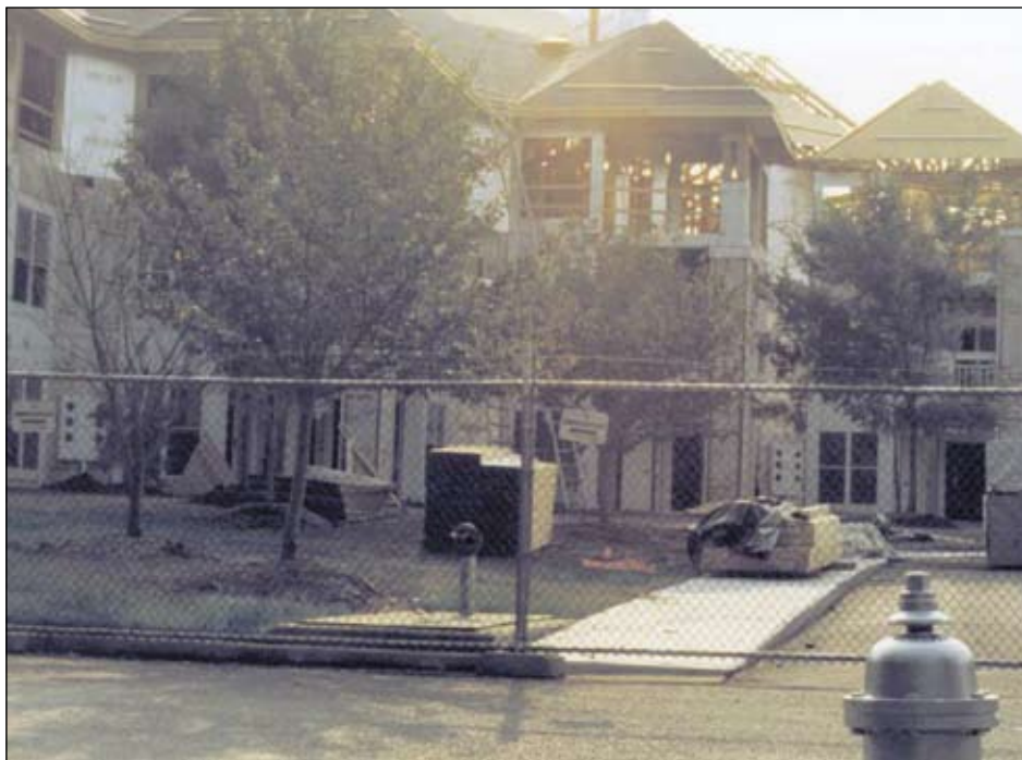
Photo 6. Fire hydrant and core siamese connection used by Engine 54 on arrival. Repairs and reconstruction are being made to the front wing; this side is the patio/balcony for each apartment.
