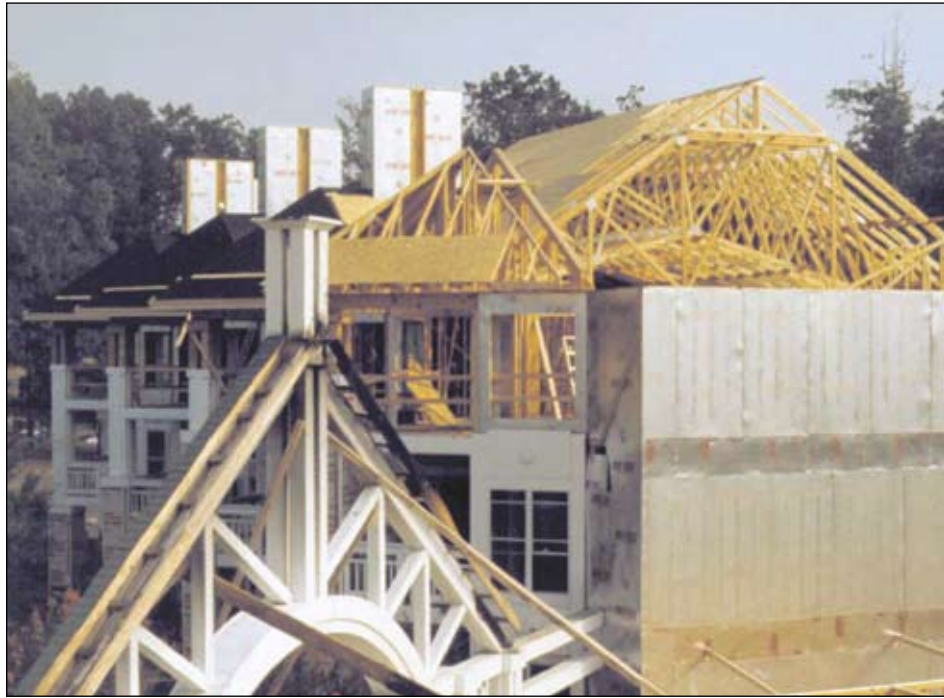
Photo 7. The remains of the front archway and the repairs and reconstruction underway for the wing in Photograph 6. The attic trusses and exterior sheathing materials are illustrated.
