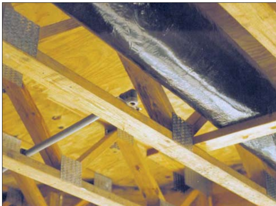
Photo 12. The parallel cord wood floor trusses used in the original construction and a polybutylene automatic sprinkler line.
