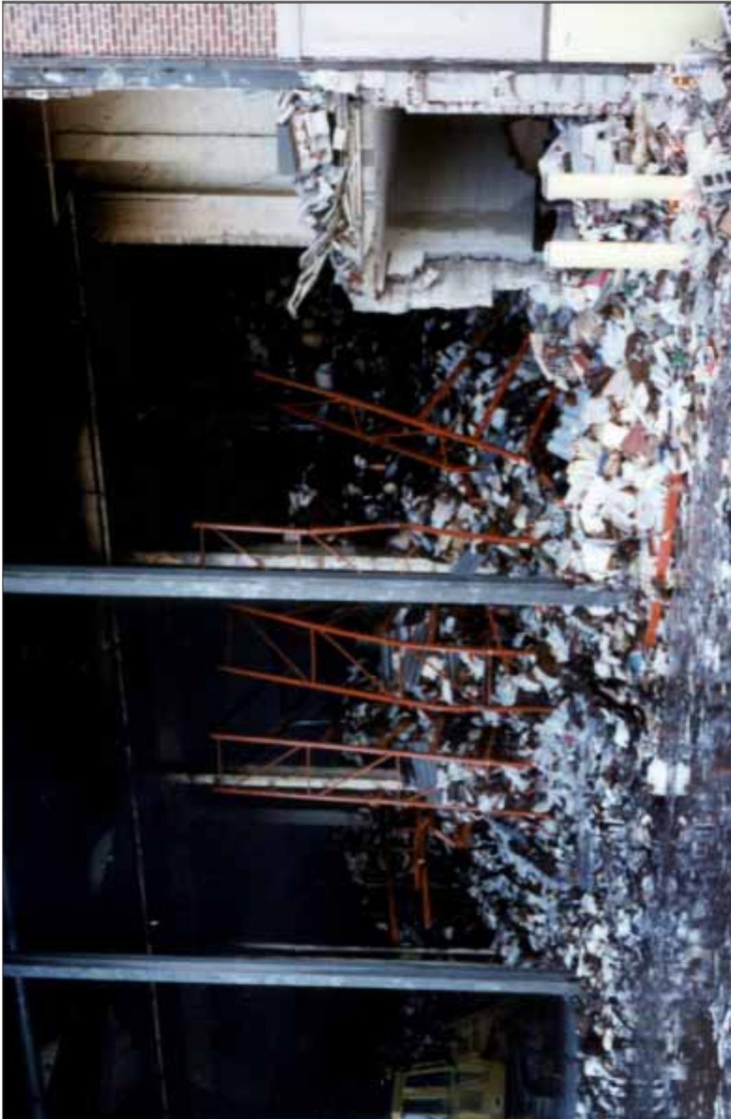
Photo 2. Typical of the rack collapse, record box failure, and documents filling the aisles. The brick-faced, hollow concrete block front wall was removed on the night of the fire.
