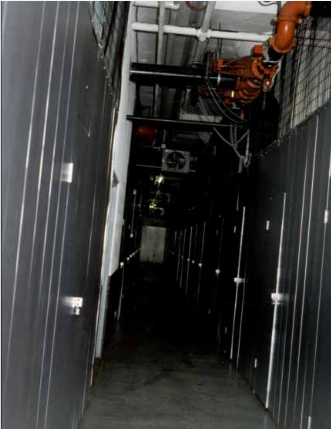
Photo 9. Typical public storage rooms or lockers located on the floor above the fire. Note the automatic sprinkler control valves and flow switch located at the ceiling level and the eight feet high solid walls topped by heavy wire mesh.
