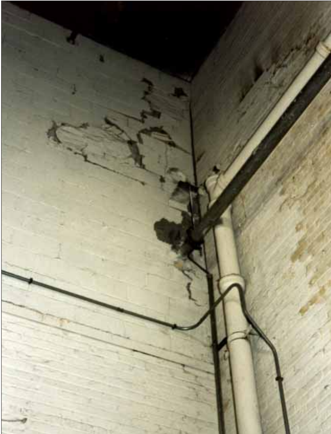
Photo 7. Masonry wall damage in Building II, north of the fire building, due to expansion of the fire wall between buildings. This corner is the southeast corner of Space 6.
