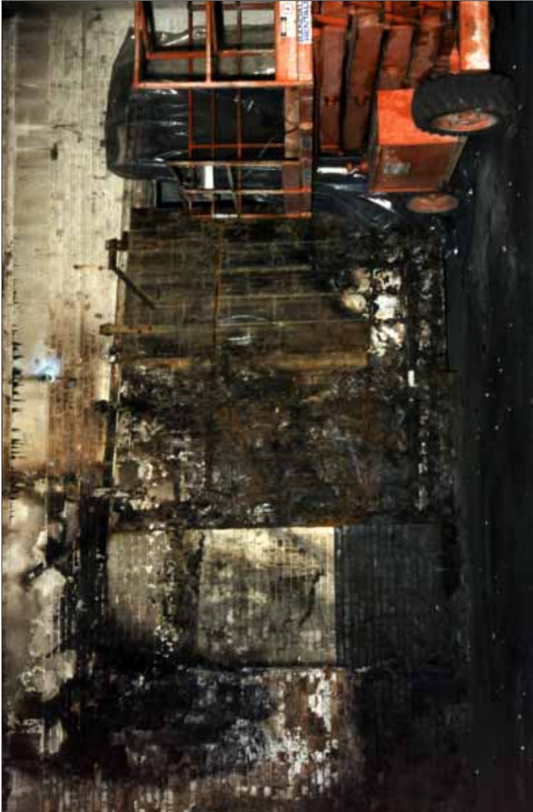
Photo 8. The fire side of the metal clad sliding fire door between Buildings III and IV. This door was supported by fire companies operating from the non-fire side of the door.
