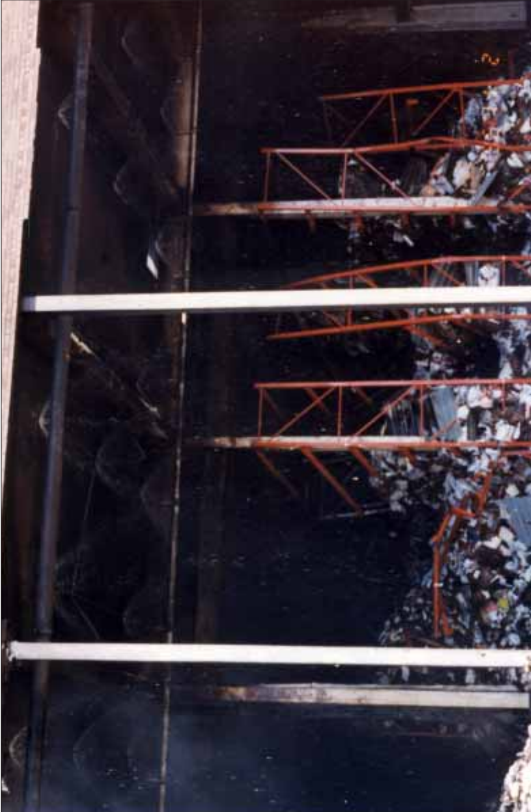
Photo 3. Racks and operating overhead automatic sprinklers near the northwest corner of Building III. Complete and partial collapse of the storage racks, shelves, and contents.
