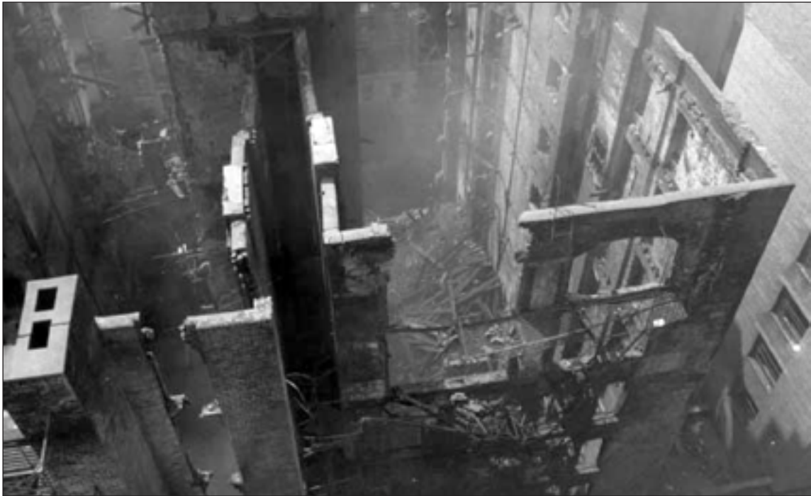
Photo 9. The Clark Building during demolition as viewed from the rear to the front.
